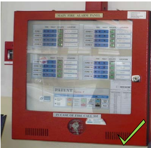
Operational ready fire alarm panel with key in break glass panel
