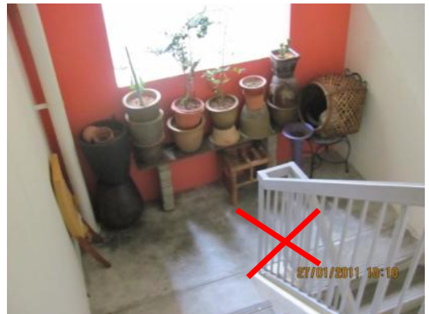
Obstruction to means of escape (staircase)
