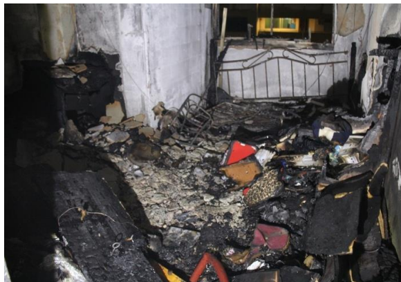
Figure 18. The contents of the room were damaged
