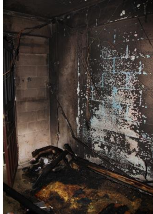
Figure 17. The burn patterns were consistent with fire origin near the main door where the battery of an electric bicycle was being charged. ▶
