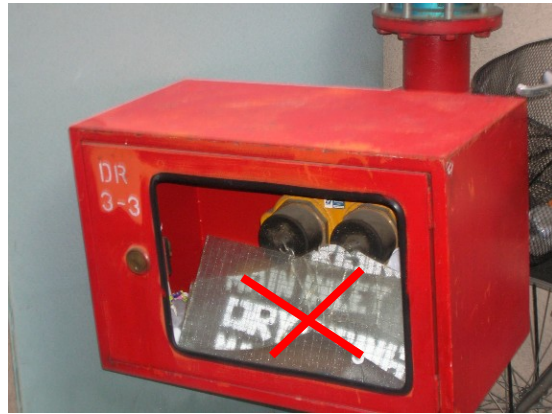
Non maintenance to the breaching inlet cabinet
