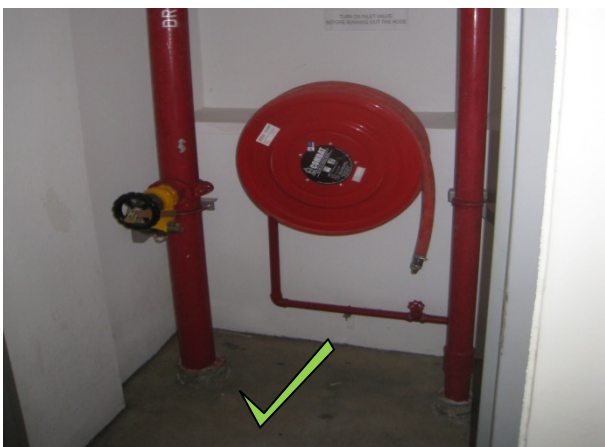
No obstruction to hosereel within hosereel compartment
