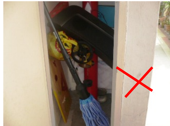
Excessive storage within dry riser compartment
