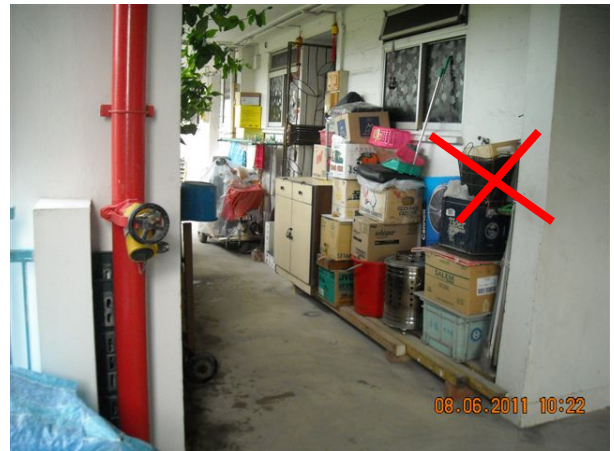
Excessive storage of combustibles
