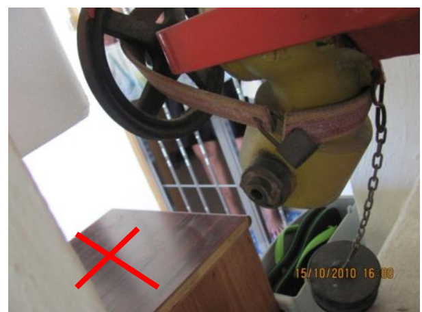
Obstruction to landing valve and missing landing valve lug
