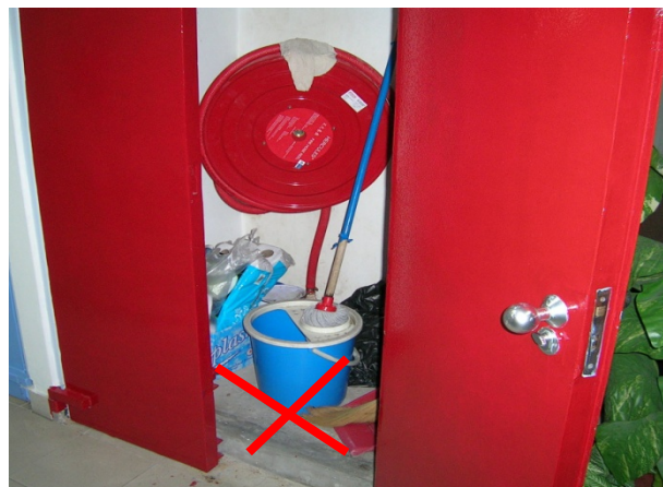
Storage of items within hosereel compartment
