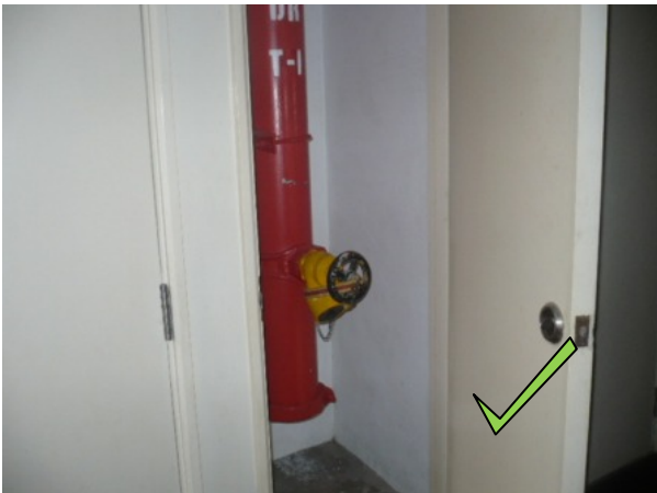
No storage within dry/wet riser compartment
