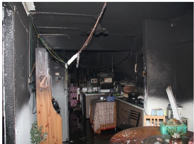
Figure 21. Other parts of the residential unit sustained heat and smoke damage
