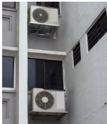
Figure 3. Condensing Units on brackets
