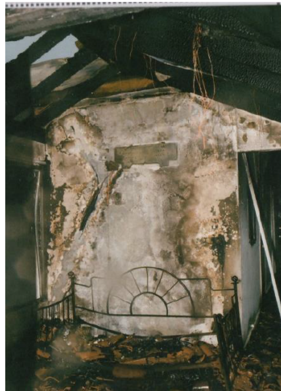
Figure 15. Another room on level 2 that was gutted by the fire
