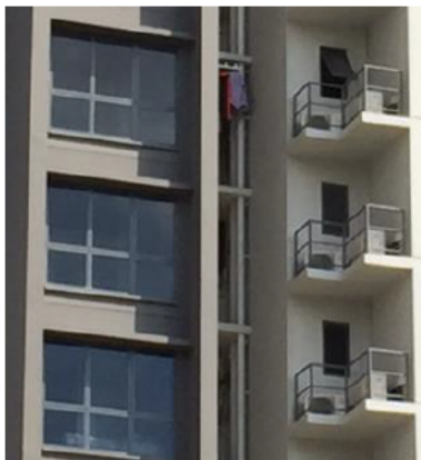
Figure 2. Condensing Units on A/C ledges
