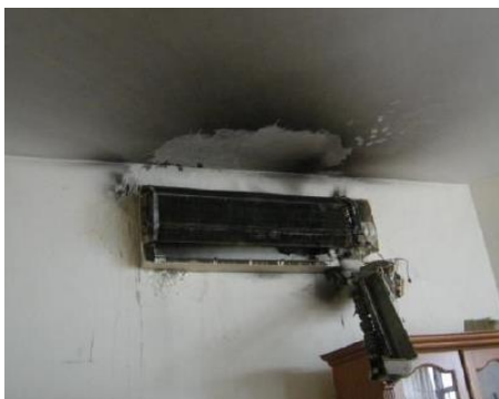
Figure 22. A localised FCU fire
