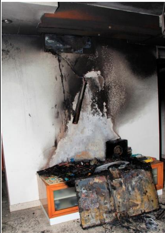
Figure 18. Drop down from the FCU fire damaged the TV and other items beneath
