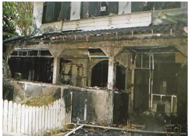
Figure 17. Other parts of the building sustained heat, smoke and water damage
