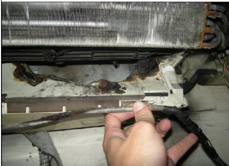
Figure 25. The burnt area on the FCU with the electrical cable that was running across
