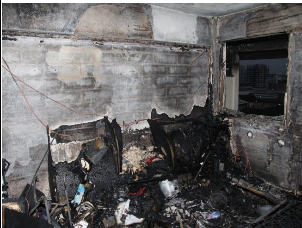
Figure 20. Fire damage was severe in the bedroom
