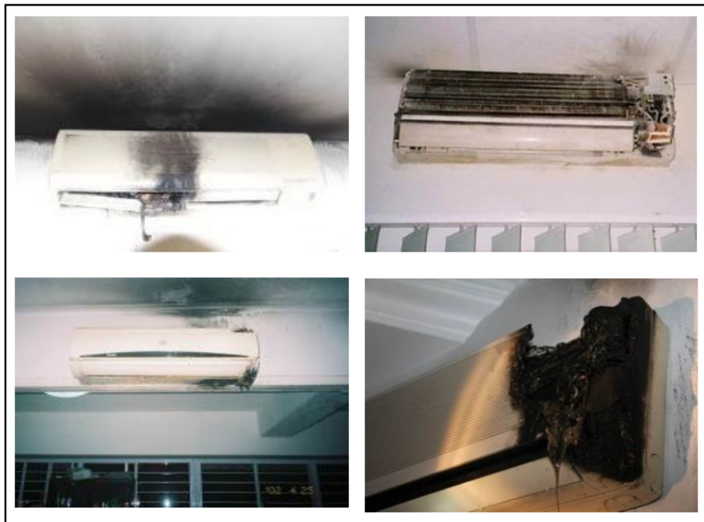
Figure 13. Localised fires involving FCUs which were on standby mode
