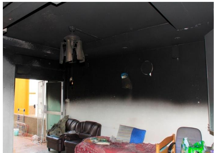
Figure 19. The apartment sustained heat and smoke damage as a result of the ceiling plume from the FCU fire
