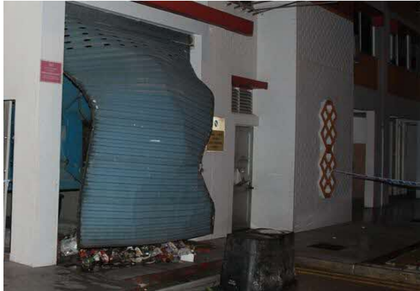
Figure 12. The roller shutter of the bin centre was observed to have bulged out
