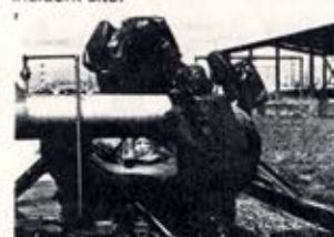
Hazmat Incident Team (HIT) mitigating a leak from a transfer pipe.
