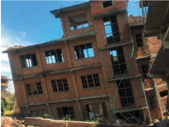
Partially collapsed building where rescuers retrieved the body of one victim
