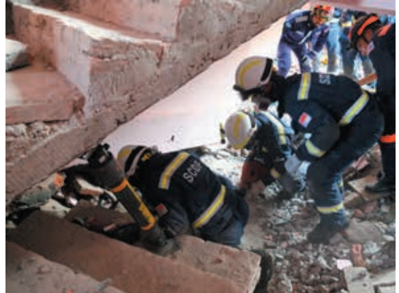
A hydraulic strut is used to support an overhanging slab of concrete stairs. Beneath it, rescuers break away concrete with an electric tool to gain access to the body
