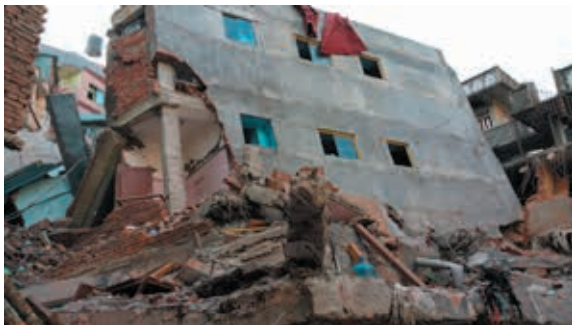
Fig.2 Collapsed entrance of a 7-storey hotel (New Star Guest House)
