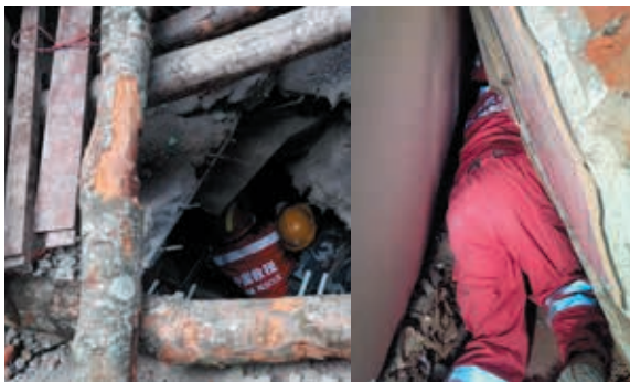
Fig.9 (a) and (b) Vertical and horizontal accesses created in the first plan
