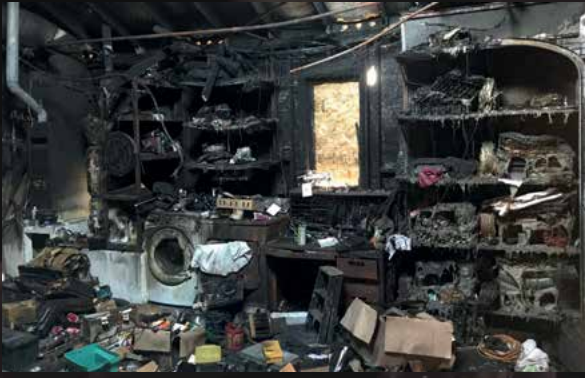
Residential garage fires typically consume large quantities of plastics, PVC and synthetic materials
