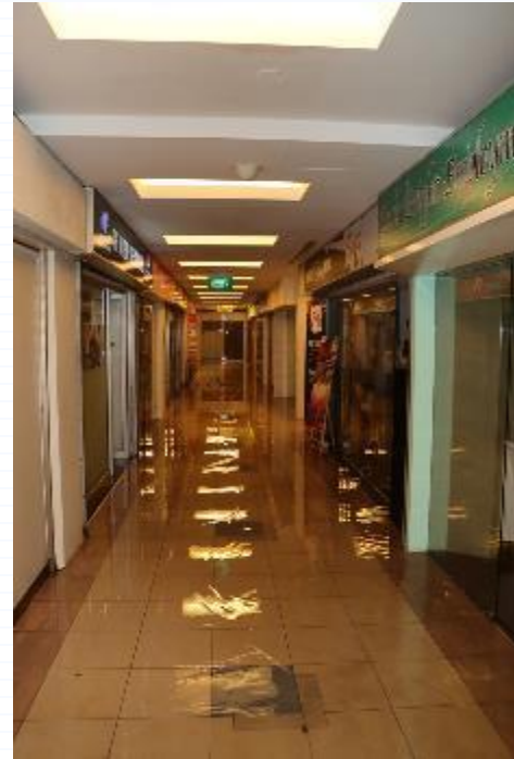
Reference photo of water damage caused by sprinkler system, courtesy of SCDF
