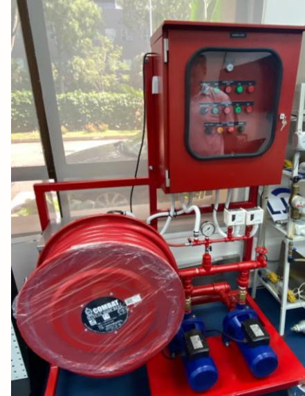
Fire Pump System
