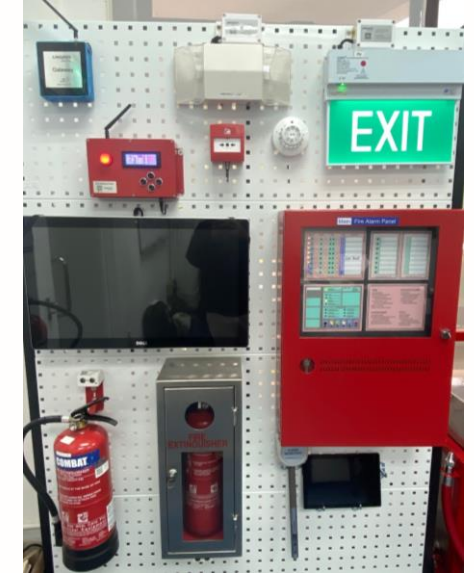
Fully Integrated Cloud-Based IoT Fire Safety System
