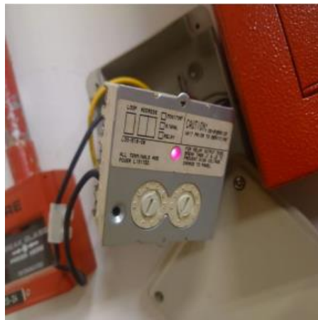
Lift – signal relay
