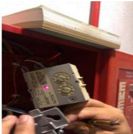
Alarm bell – signal relay
